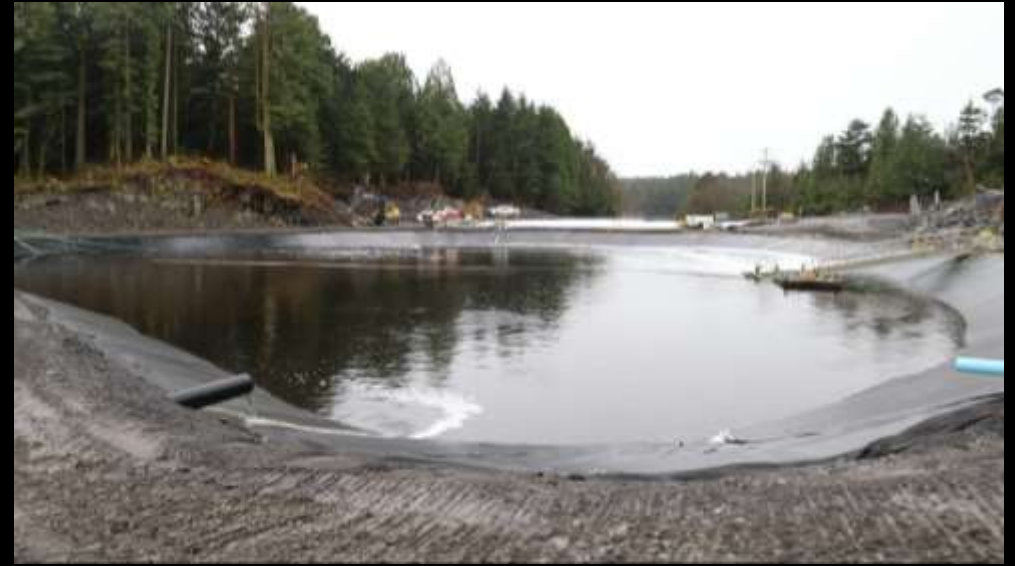
Pictured above: Image of the landfill lagoon while it was still under construction
