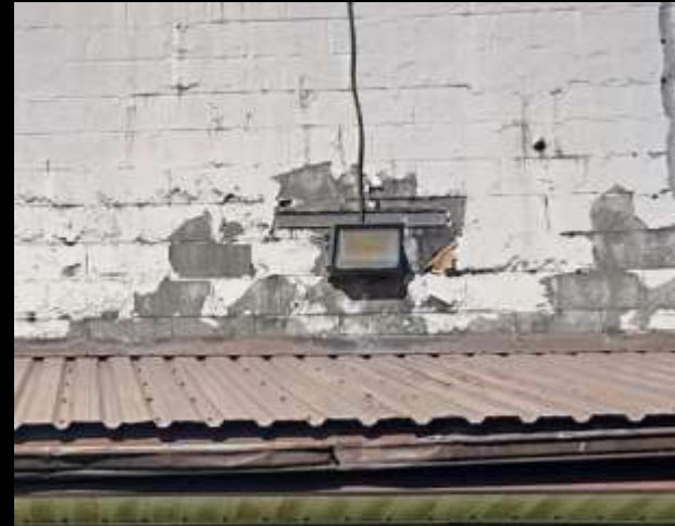
Pictured left: Deteriorating conditions of the exterior of the Rec Centre is apparent
