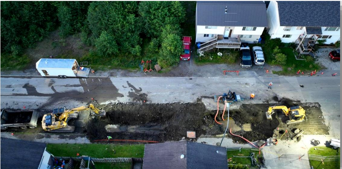
Pictured above — replacement of the full length of waterline under 7th Avenue East is one of the proposed capital projects for 2024. pending Federal funding approvals.
