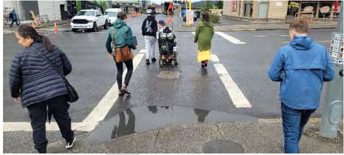
An intersection with poor drainage
