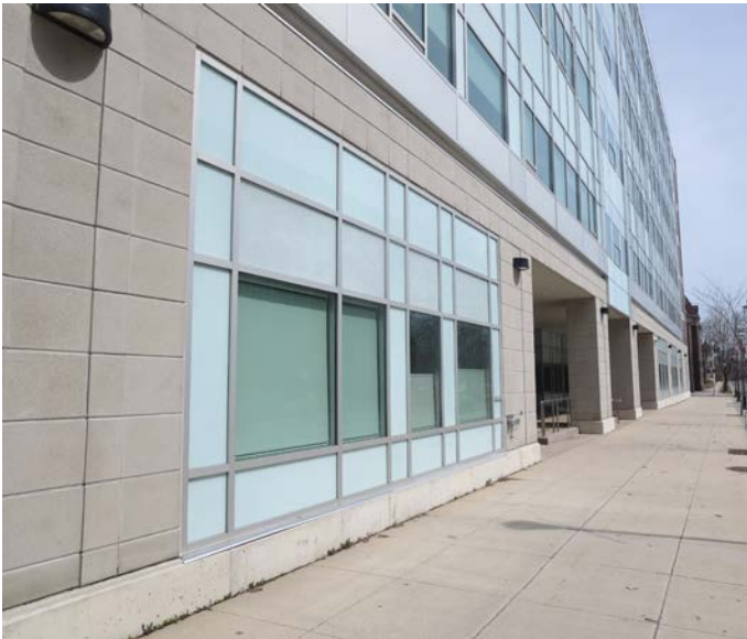
This building is not well articulated. The facade is flat and planar. Datum lines are weak; those between ground floor and upper storeys do not have good continuity.
